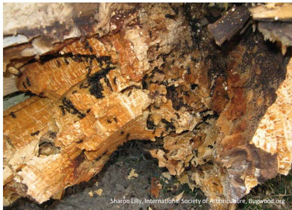
Fig. 1: Carpenter ant colony in wooden beam
