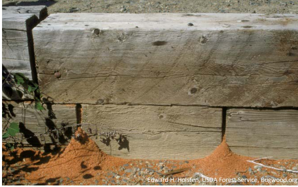
Fig. 6: Sawdust ‘dumps’ – evidence of carpenter ant activity
