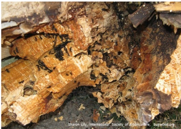
Fig. 1: Carpenter ant colony in wooden beam
