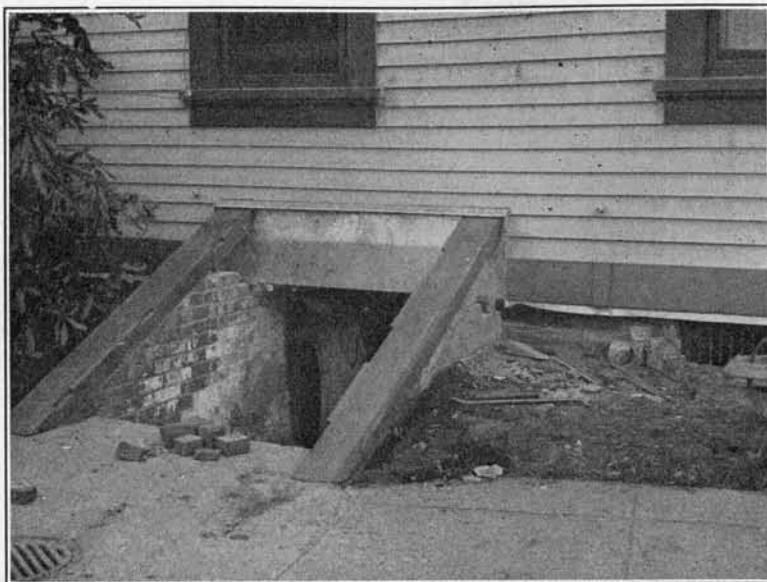
FIGURE 6. Installation of a metal termite shield in an infested house. Susceptible cellar hatching shielded from the building.
