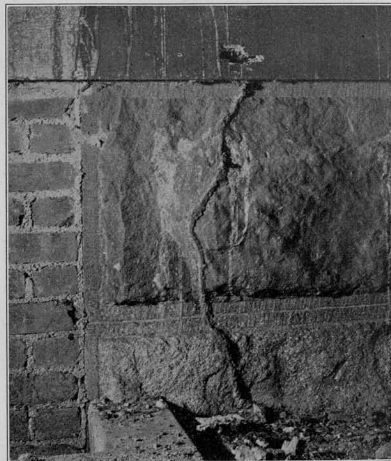
FIGURE 5. Termites constructed this shelter tube from wood to the ground in a partly excavated area (formerly exterior).
