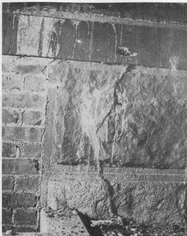
Figure 2. Termites constructed this shelter tube from wood to the ground in a partly excavated area, formerly an exterior wall.
