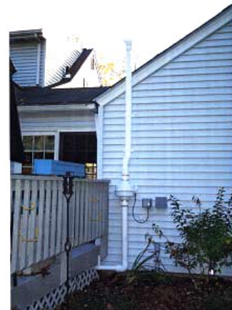
Depressurization System Vent Pipe Outside Home
