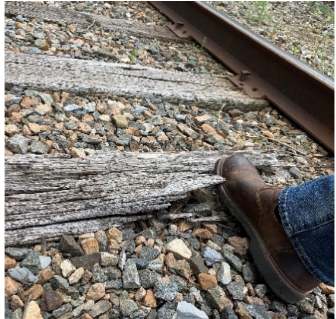
Figure 13 Wooden Ties with Severe Rotting
