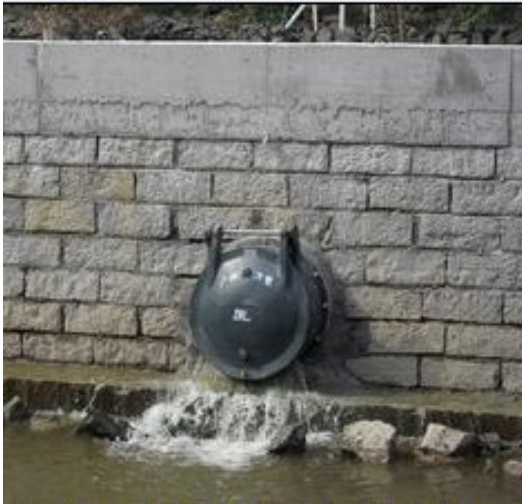
Stormwater Flap Gate
