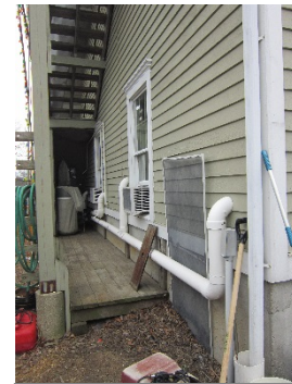
Elevated Pipes 5 Green Hill Place
