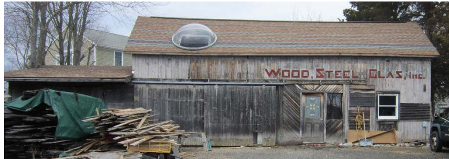
9 Old Post Road Note stains from flooding, opening in sliding garage door, elevated utility to the right.
