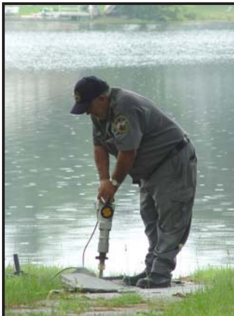
Correctional Plumber Carlos Desousa breaks up the cement around the Shaker tombstones.
