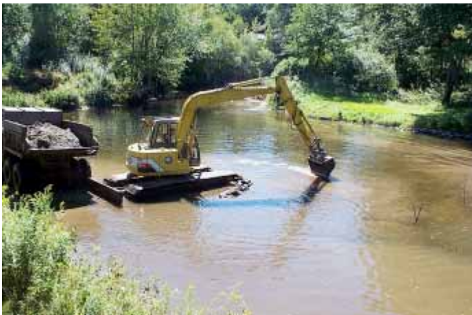
A special, low ground pressure excavator digs a deep pool area in the Hop River to create habitat for fish.
