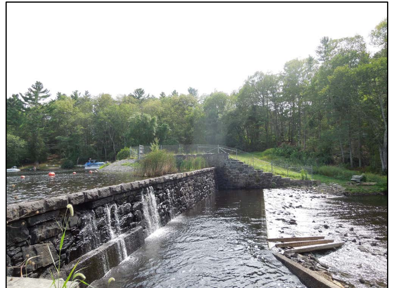
Pachaug Pond Dam
