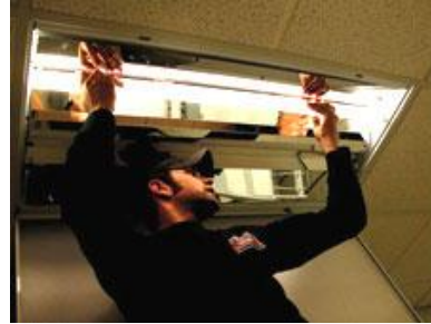
Retrofit Projects & Small Business
