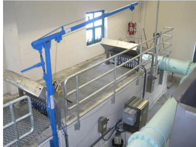
UV disinfection system
