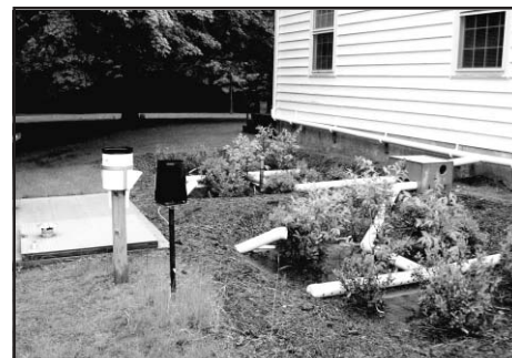
Influent is piped to rain garden from building roof
