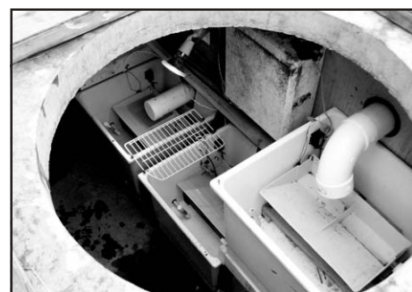
Effluent is collected and monitored in subsurface pump chamber
