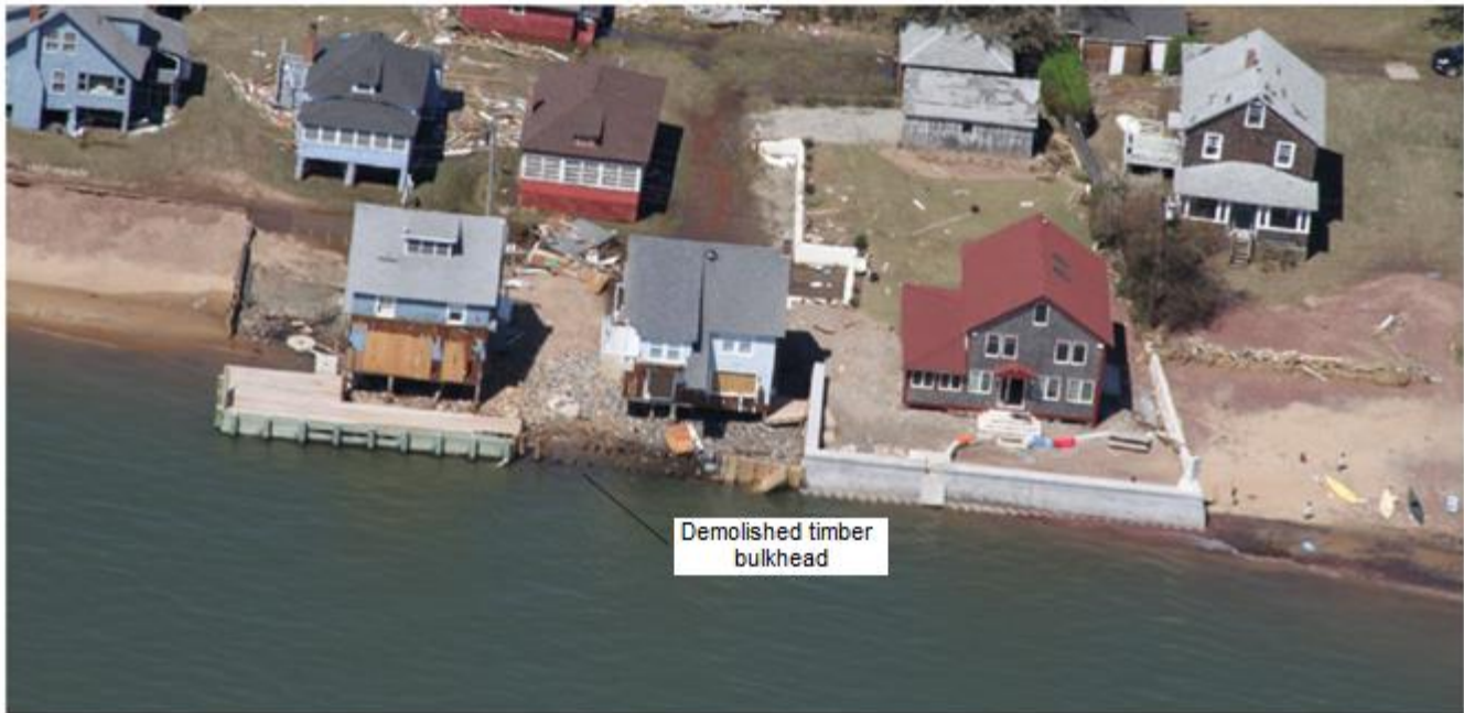
Figure 2. Photo of coastal storm damage taken by DEMHS on 08/30/2011 following Tropical Storm Irene
