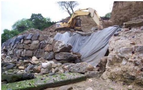
Unauthorized seawall under construction Shippan Point, Stamford Photo Credit: DEEP OLISP
