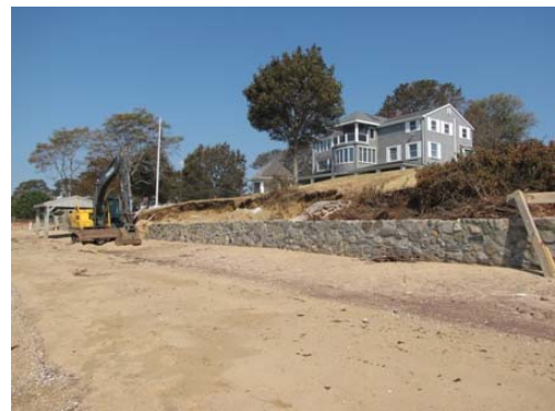
Erosion behind a seawall in Madison resulting
