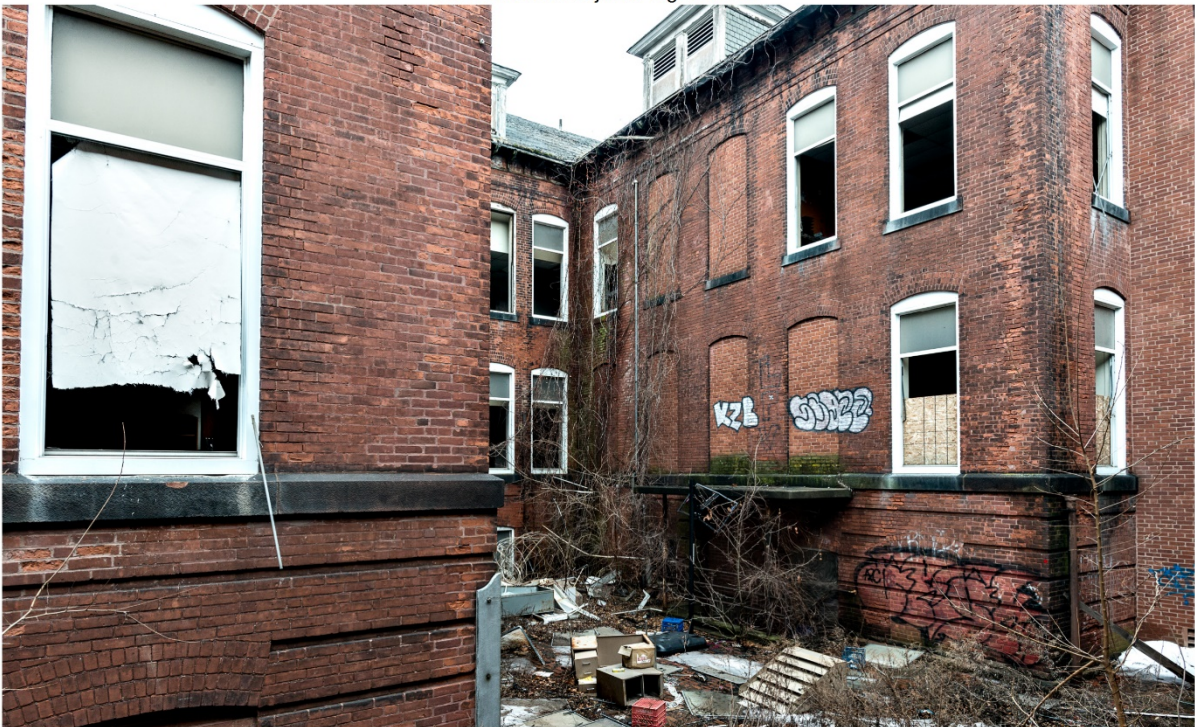
Photo 4. View northeast showing south elevation of elementary school from junior high school auditorium.
