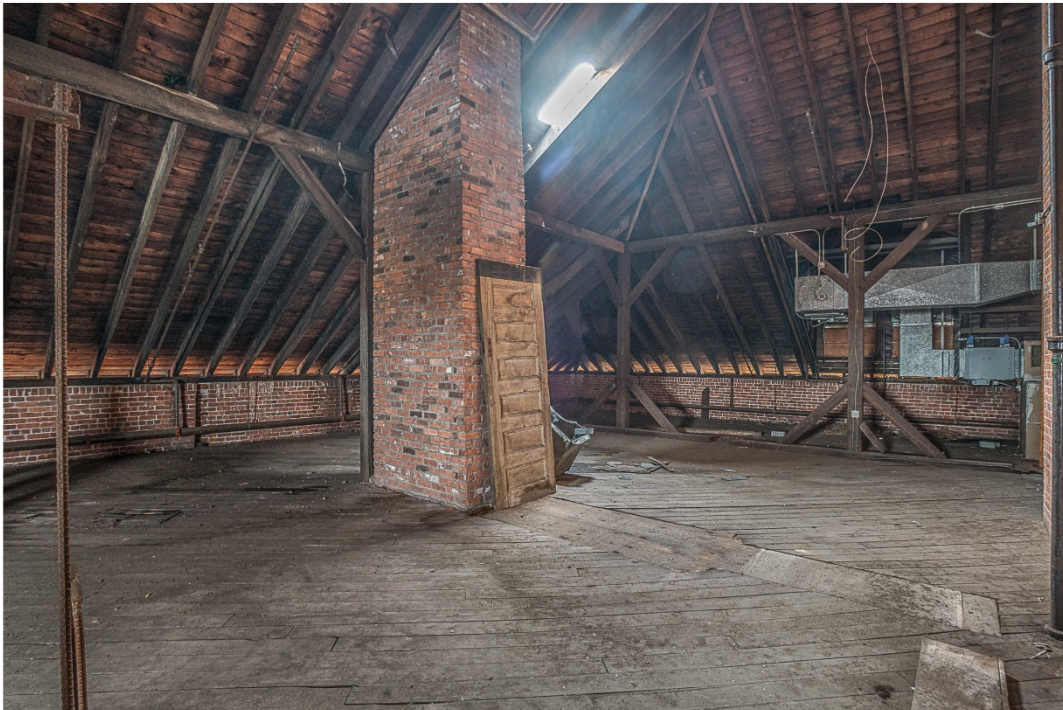
Photo 18. Interior view southwest showing wood floor, brick knee walls existing skylight and exposed wood structure in attic of elementary school.
