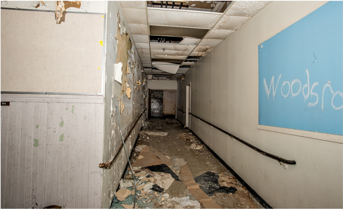
Photo 13. Interior view south showing connecting corridor from elementary school to junior high school.
