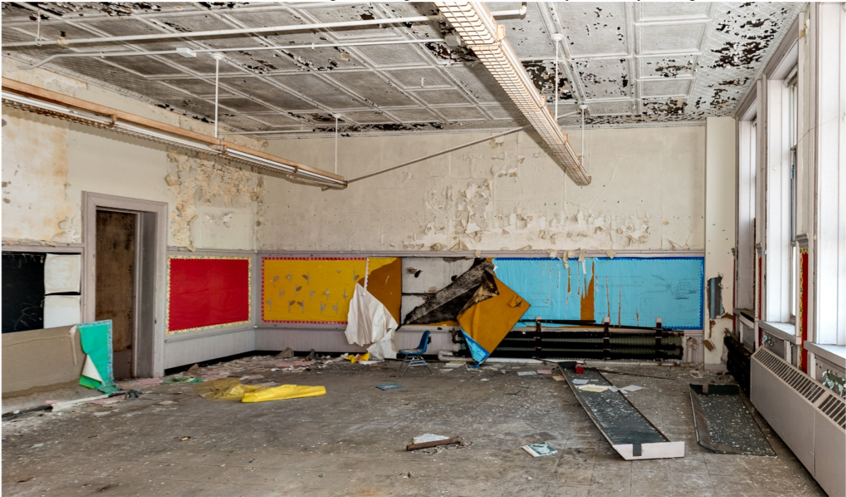
Photo 14. Interior view southwest showing original paneling, moldings, plaster walls, flooring, stamped metal ceiling and blackboards in typical classroom on north side of elementary school.
