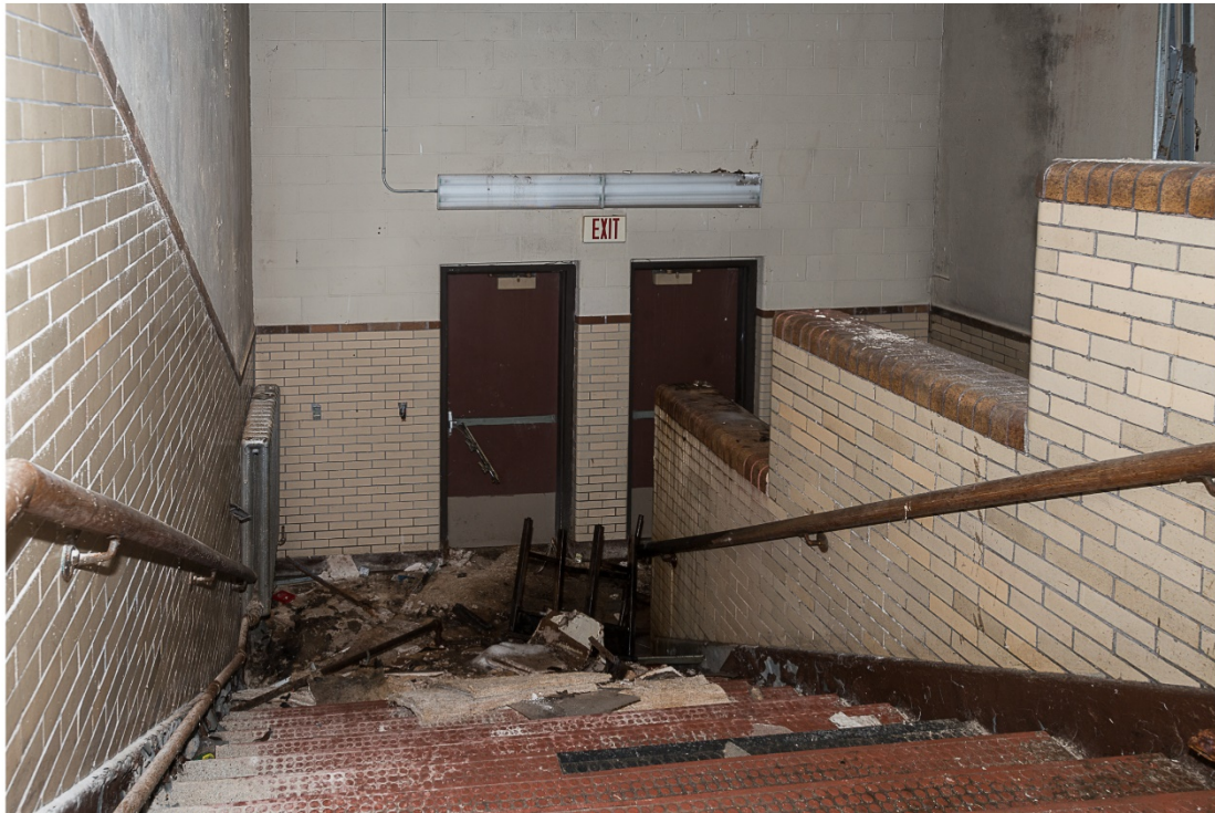
Photo 20. Waltersville School. Interior view east showing east entry stairway of junior high school. .
