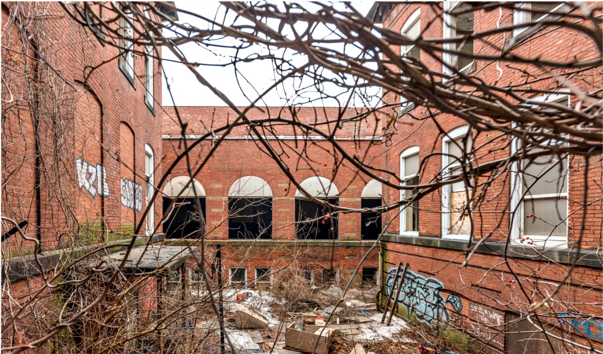
Photo 10. View south showing east and west elevations of elementary school south wings, as well as part of north elevation of junior high school.
