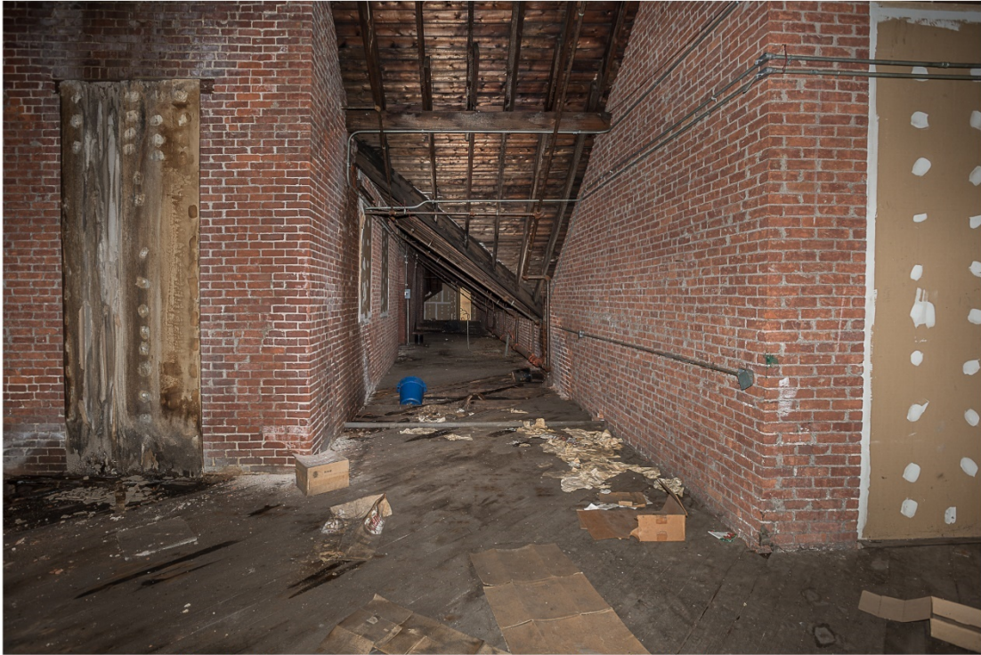
Photo 17. View west of attic corridor showing wood floor, brick walls and rafters.
