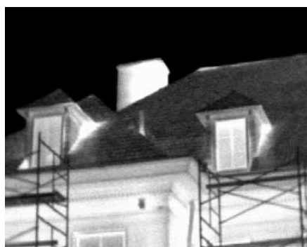
Fig. 1. Infrared thermograph of a building eave area of Oldfields, Indianapolis Museum of Art, Indianapolis, showing warm surfaces (light) and cold spots (dark). The attic floor is insulated, and the walls are not. The walls were in good condition despite high indoor humidity. Courtesy of the Hillier Group.
