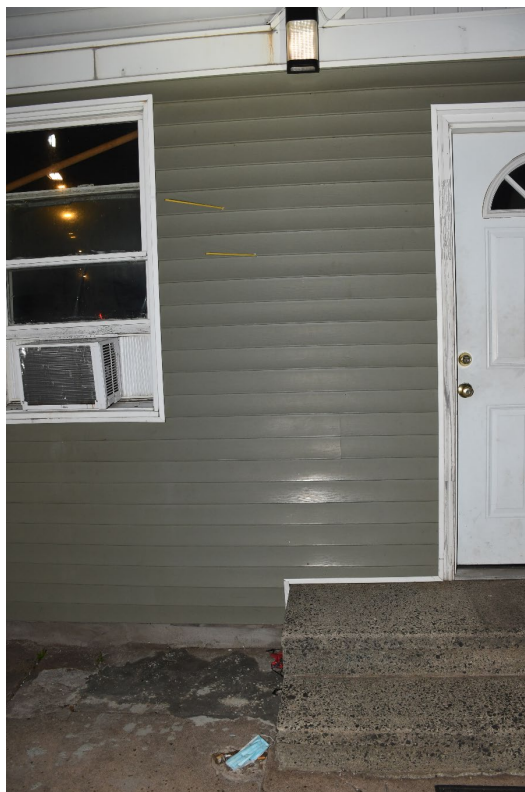
[Trajectory rods showings bullet holes in siding of 167 Chapel Street]
