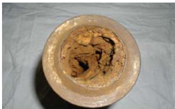
This view shows the female end of the pipe, which was attached to the riser at an upper floor. It is almost completely obstructed with rust, scale, and debris
