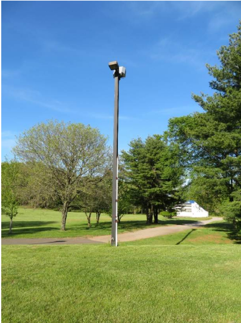
Photo 1: Sample photo illustrating the existing light pole.
