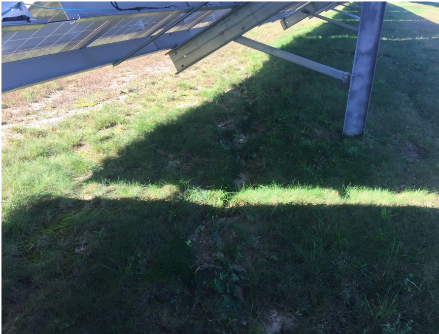
Figure 1 - Eroded path of concentrated Flow from runoff off solar panel (East Lyme)
