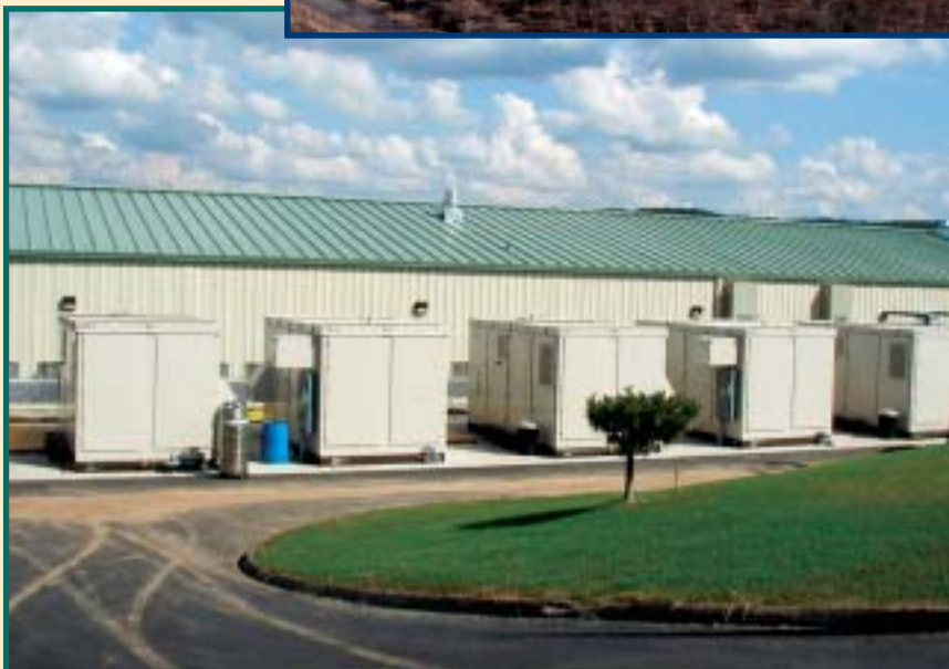
1.2 MW of fuel cell capacity at the Connecticut Juvenile Training Center, Middletown
