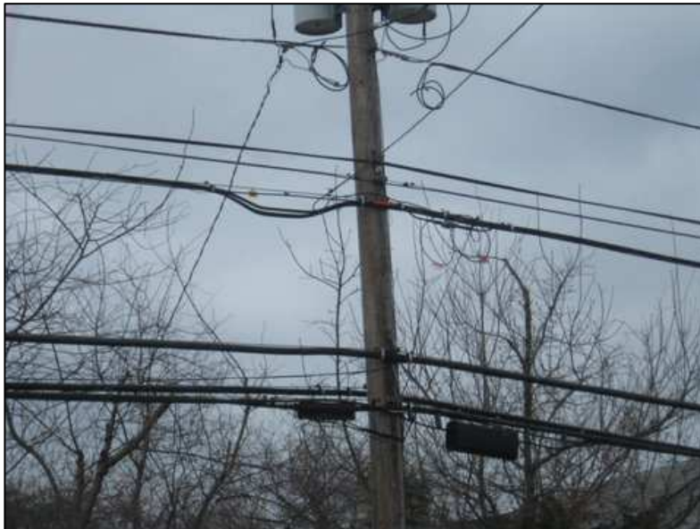
Typical Splice Enclosures. Typical splice enclosures used by the utility company (on the bottom cables) that are similar to the fiber splice enclosures that would be used for this project. The proposed fiber would be similar to the smaller cables just above the bottom 2 cables.
