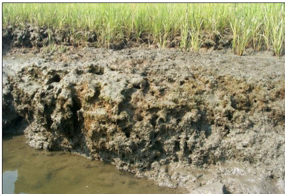
Figure 3. Erosion along the Neck River in Madison, CT (Courtesy of Peter Thiel).
