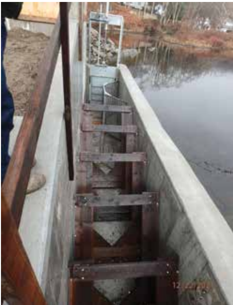
Connecticut's newest fishway is this Denil Fishway at the Upper Collinsville Dam on the Farmington River, which was completed early in 2022. It is dam #5 in the table.
