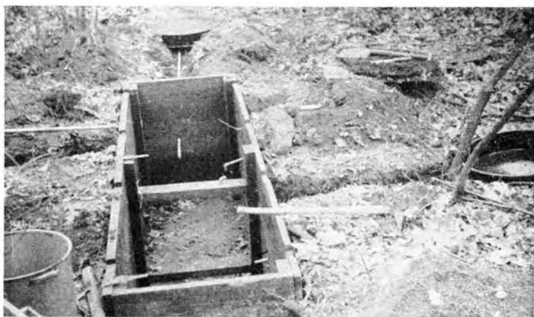
FIGURE 5. Installation of tank lysimeters. Tank No. 6 at the far end of pit; No. 3 on extreme right.
