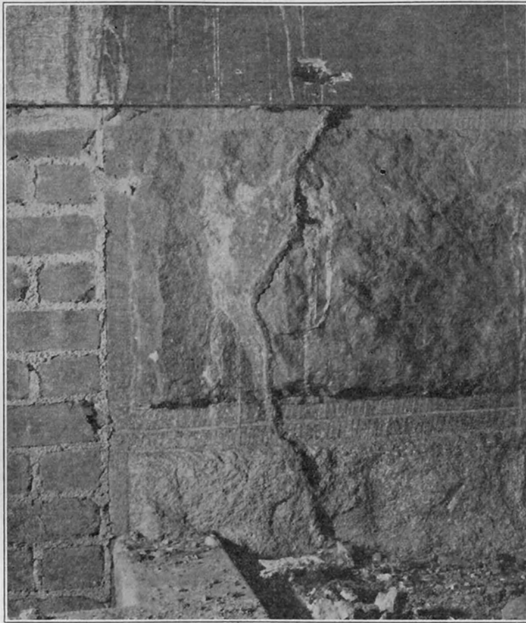
FIGURE 86. Termites constructed this shelter tube in a partly excavated area to gain entry to wood in this building.
