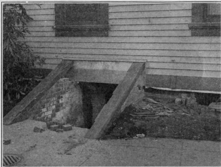
FIGURE 92. Susceptible cellar hatchway shielded from a house.
