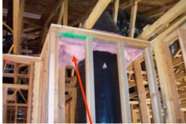
Air Sealing Installation That Will Not Comply
