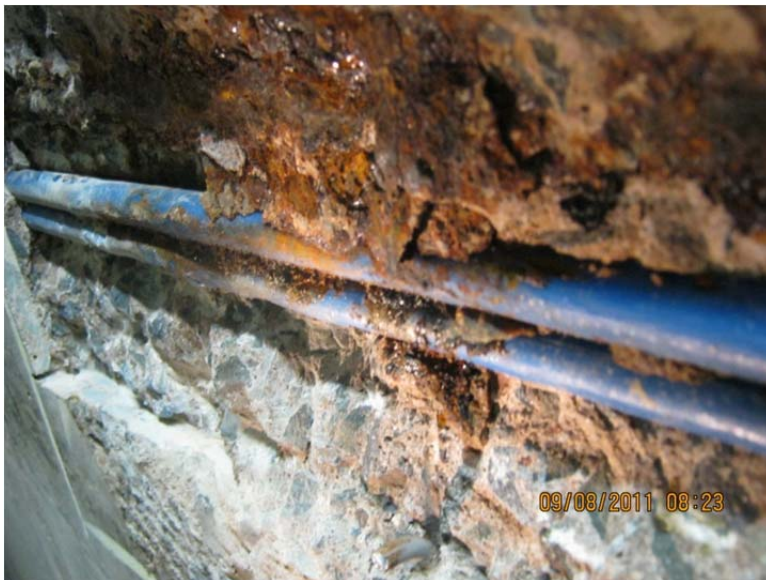
Figure 15. Corrosion damage to mild reinforcing steel and damage to sheathing on soffit.
