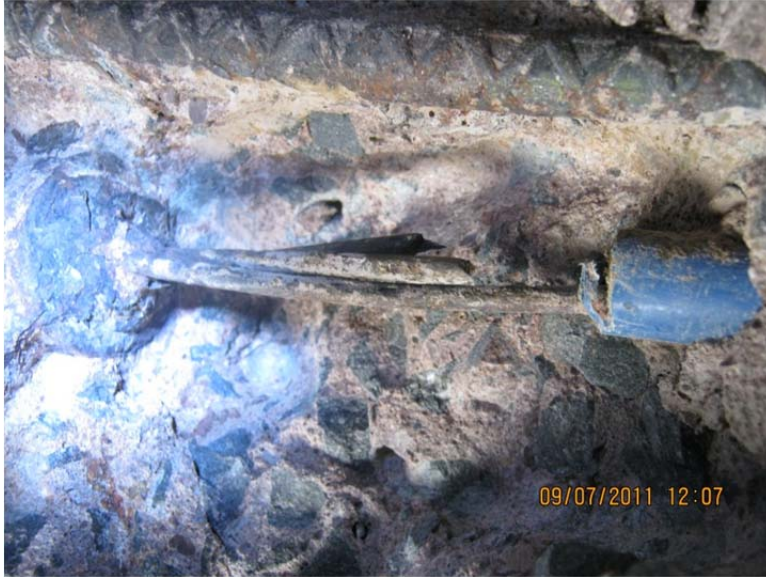
Figure 10. Failed strand at construction joint. Note corrosion on anchorage and failed wires.
