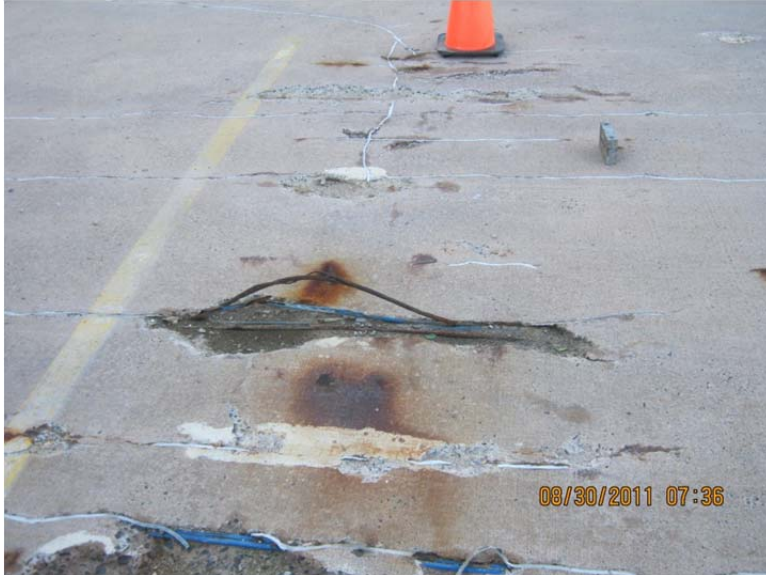
Figure 5. Failed post-tensioning on Level 6.
