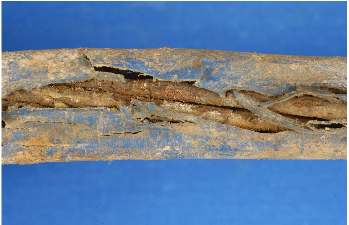
Figure 5. Close view of location shown in Figure 4. L3607 093011 05
