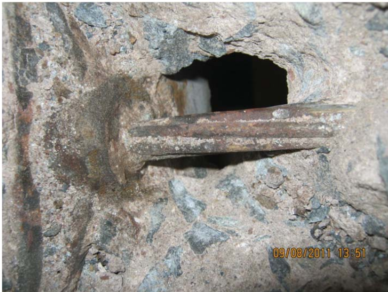
Figure 11. Corrosion damage on strand, without strand failure.
