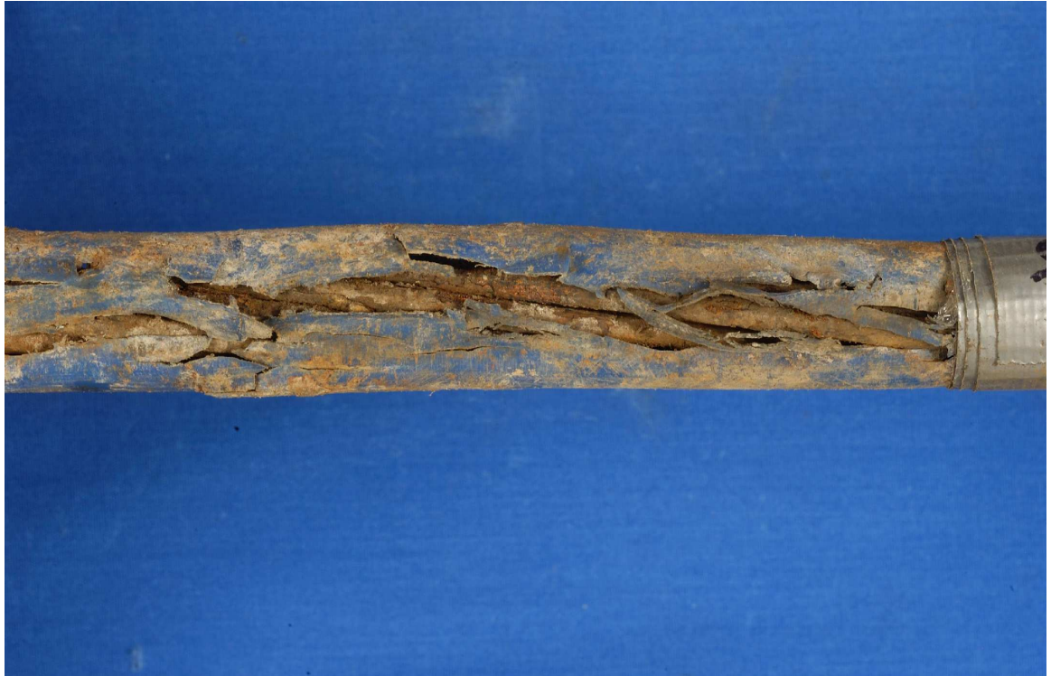
Figure 4. Severely damaged PE sheathing and visibly corroded strand wire on strand #2.
