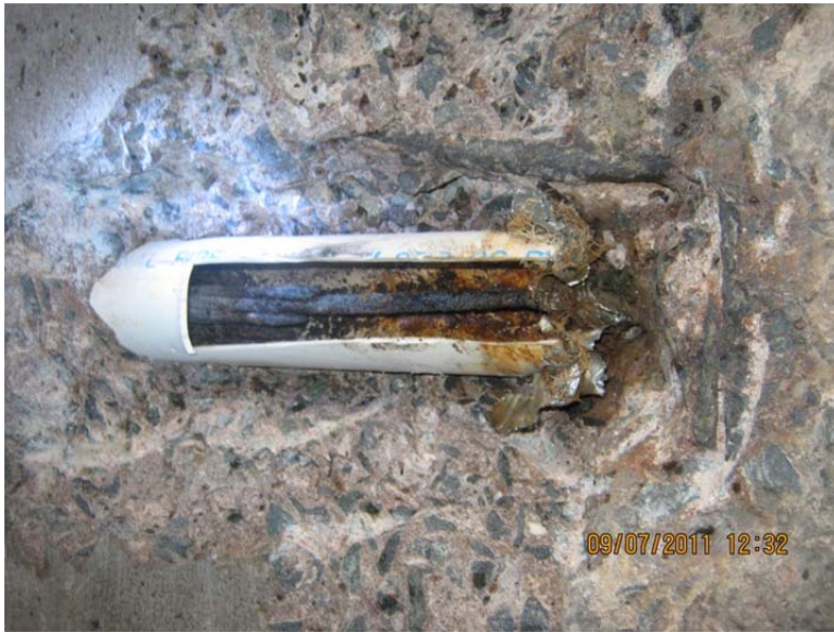
Figure 12. Failed strand at construction joint (possibly failed during original construction).
