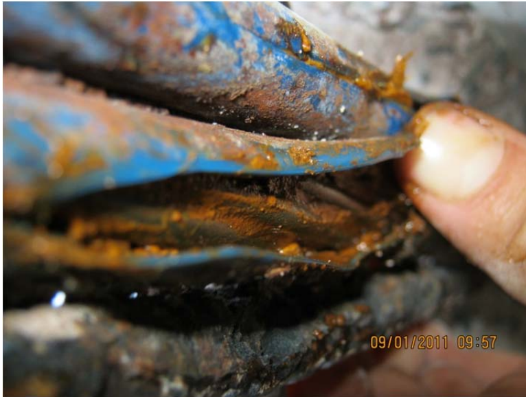
Figure 14. Water and emulsified grease on strand.
