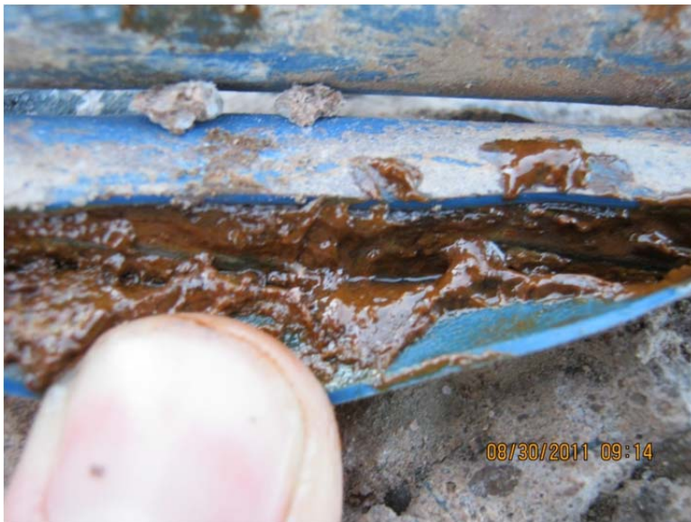
Figure 6. Emulsified grease on post-tensioning grease.
