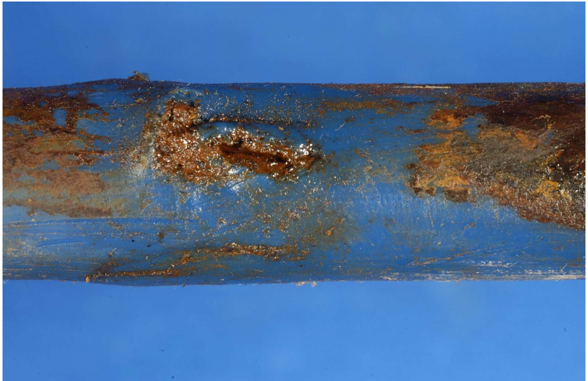
Figure 3. Second location of many on strand #1 showing evidence of sheath damage.
