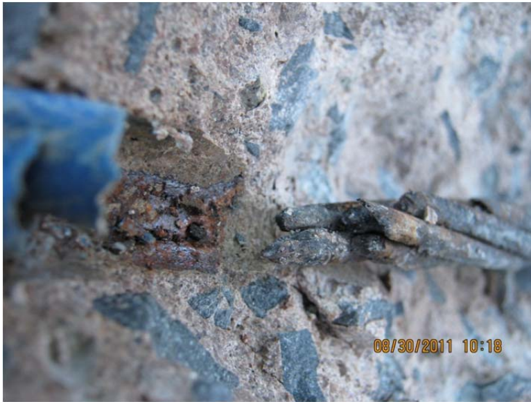
Figure 7. Brittle failure of post-tensioning strand on Level 6.
