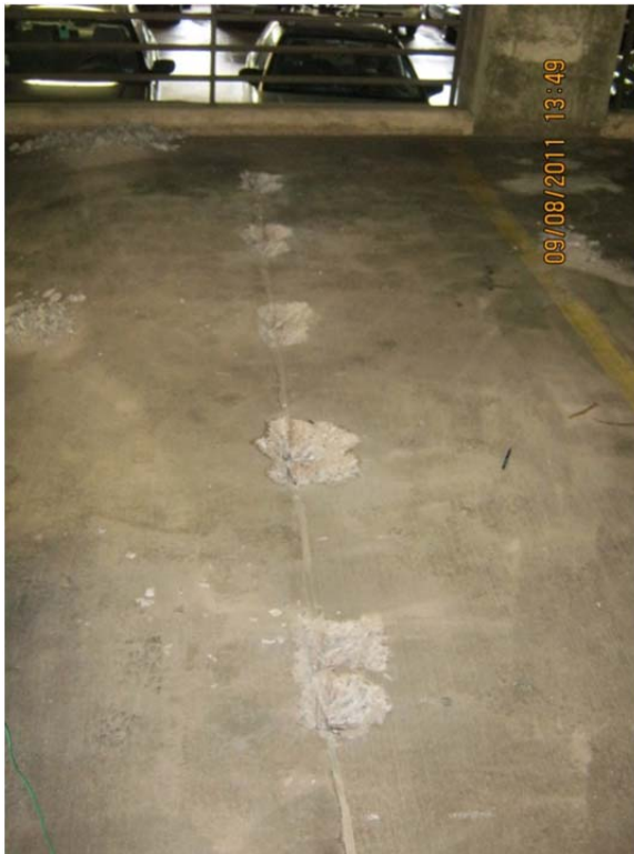
Figure 9. Openings at construction joint on Level 2.
