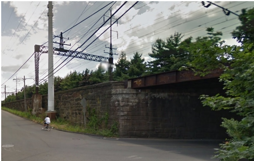
Figure 3-46—View of Fort Point Street Bridge and stone-faced abutment, looking east (from Google Maps)
