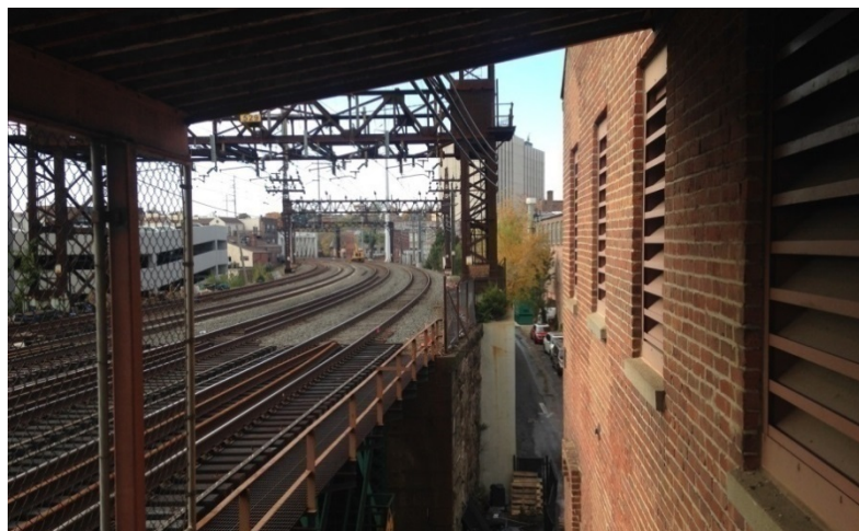
Figure 3-37—View of Walk Bridge west approach and abutment, looking west from fire escape with Maritime Aquarium on right
