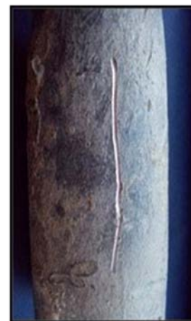
Picture of a Scratch on a Lead Service Line
