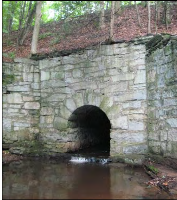
Arch-type railroad crossing (SC-02) constructed of stone and extending approximately 125 feet. The crossing may prevent fish passage and is suffering from downstream scour evidenced by the large pool shown in the photograph.
