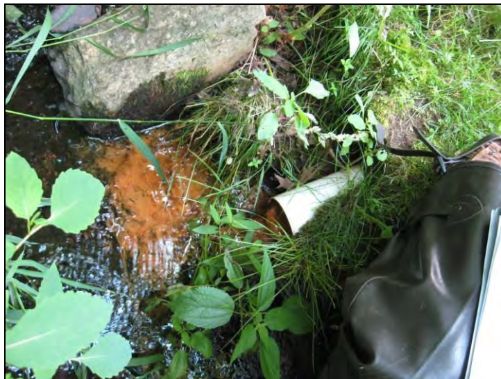
Outfall pipe originating from a residential property on the left bank of segment TB-04C.
