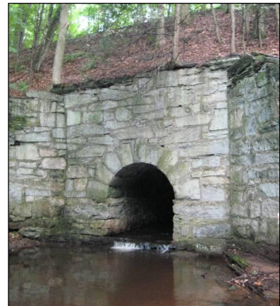
Arch-type railroad crossing (SC-02) may prevent fish passage and is suffering from downstream scour evidenced by the large pool shown in the photograph.
