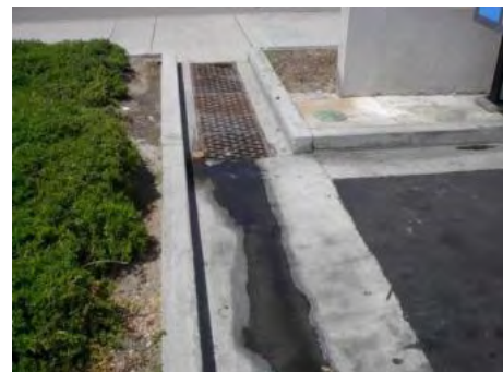
Figure 6-34. Wash water from a commercial car wash discharging down a storm drain is an example of an illicit discharge. Source: EPA
