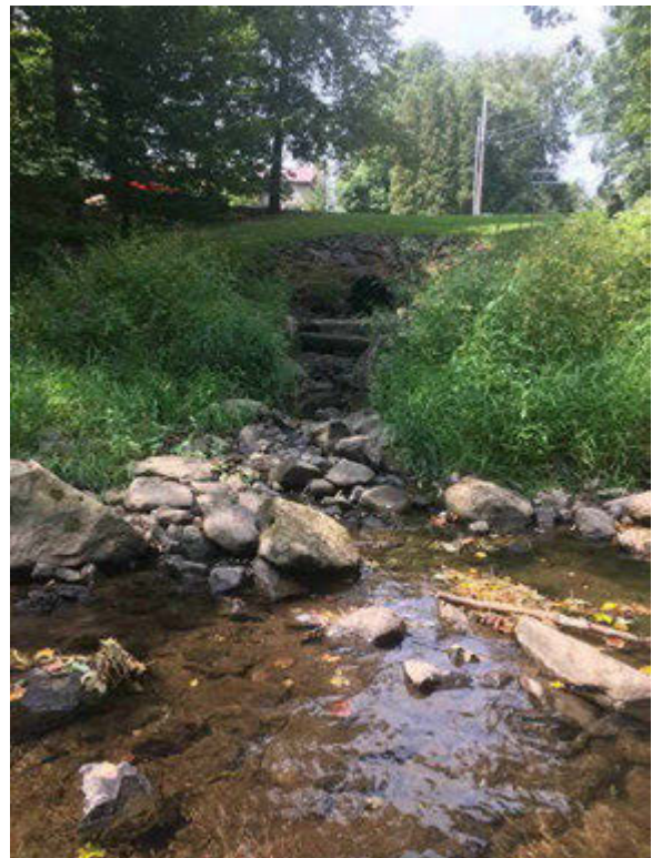
Figure 4: Stormwater outfall at head of reach Pomperaug-03.
