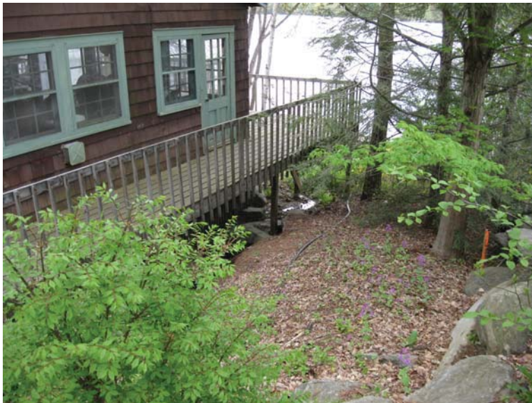
Drainage goes under existing deck & is flooding yard Insufficient room to create stabilized channel, Will require piping
