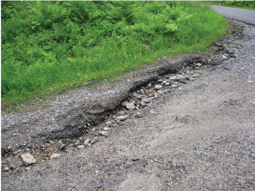
Eroded Shoulders - Install shoulder armor or create grassed swales.
