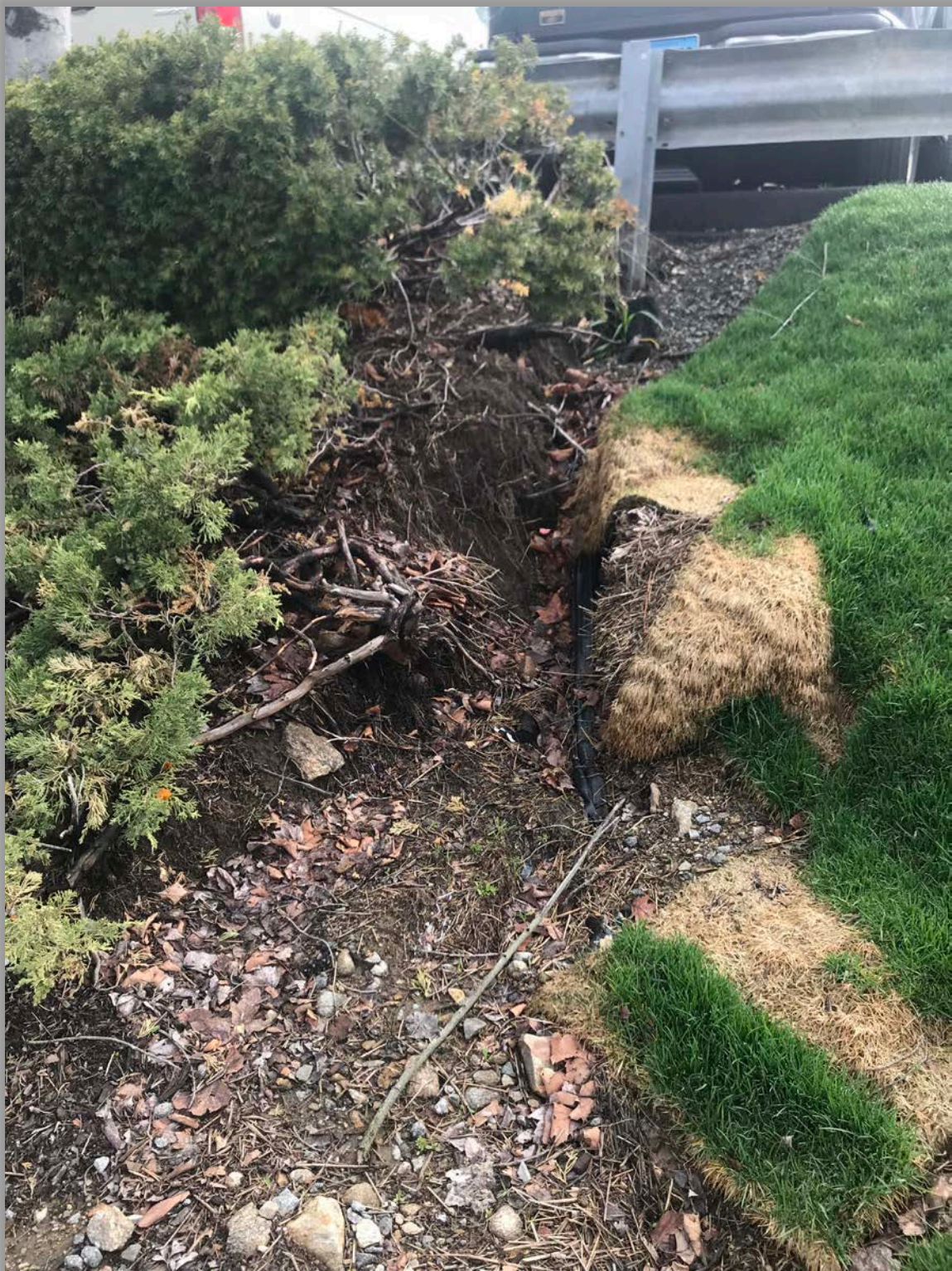
Figure 5.37: Parking lot runoff not adequately intercepted, leading to erosion
