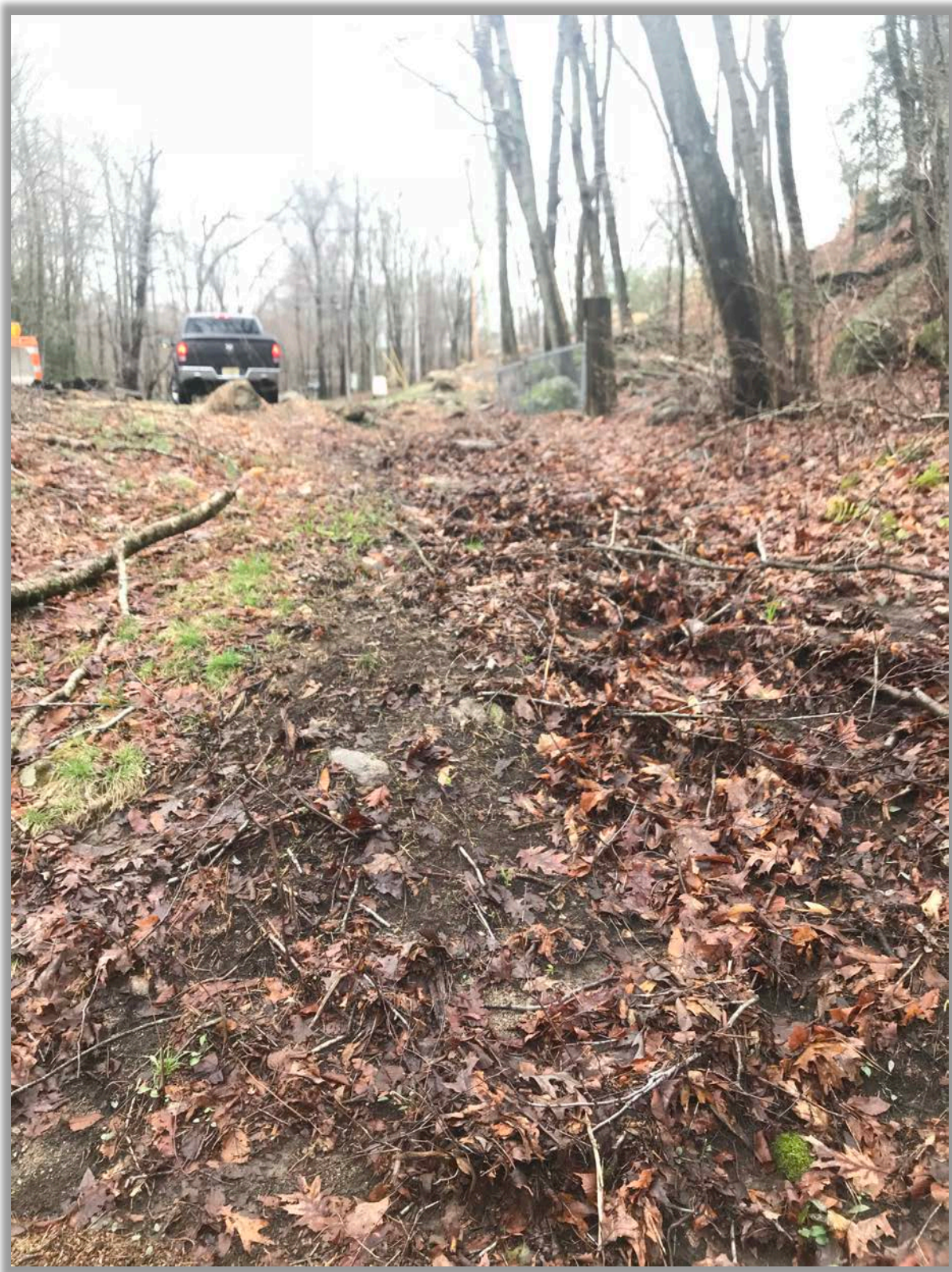
Figure 5.24: Unmanaged stormwater flow from Sturbridge Road
