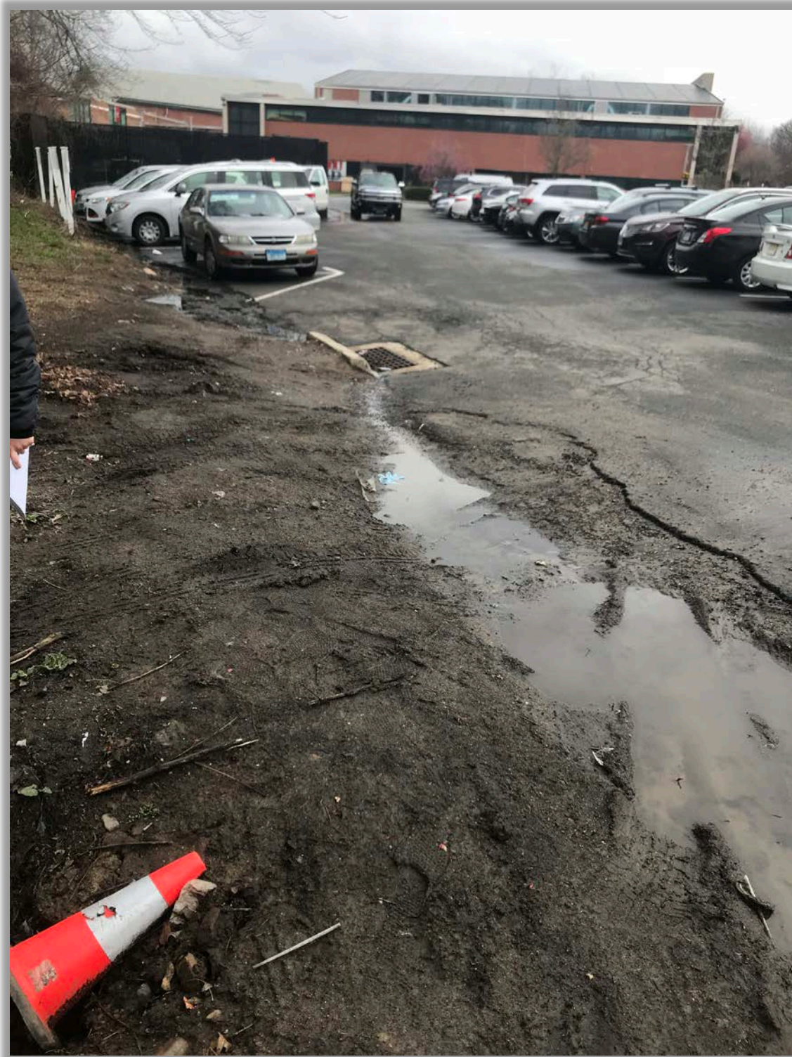
Figure 5.38: Poor stormwater management leads to ponding and generation of solids
