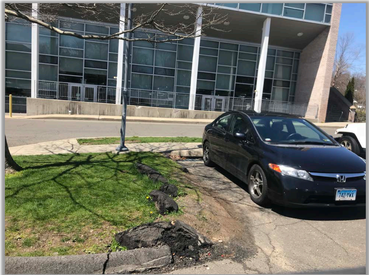
Figure 5.43: Another catch basin showing capture of leaf litter and solids from eroding lawn surface and poor state of repair for curbing
