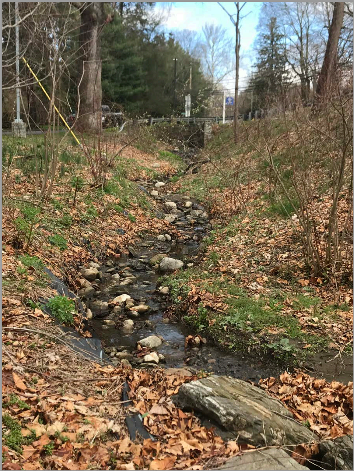
Figure 5.27: Candidate site for step bioretention system to manage stormwater conveyance and improve channel stability; geotextiles from previous stabilization exposed
