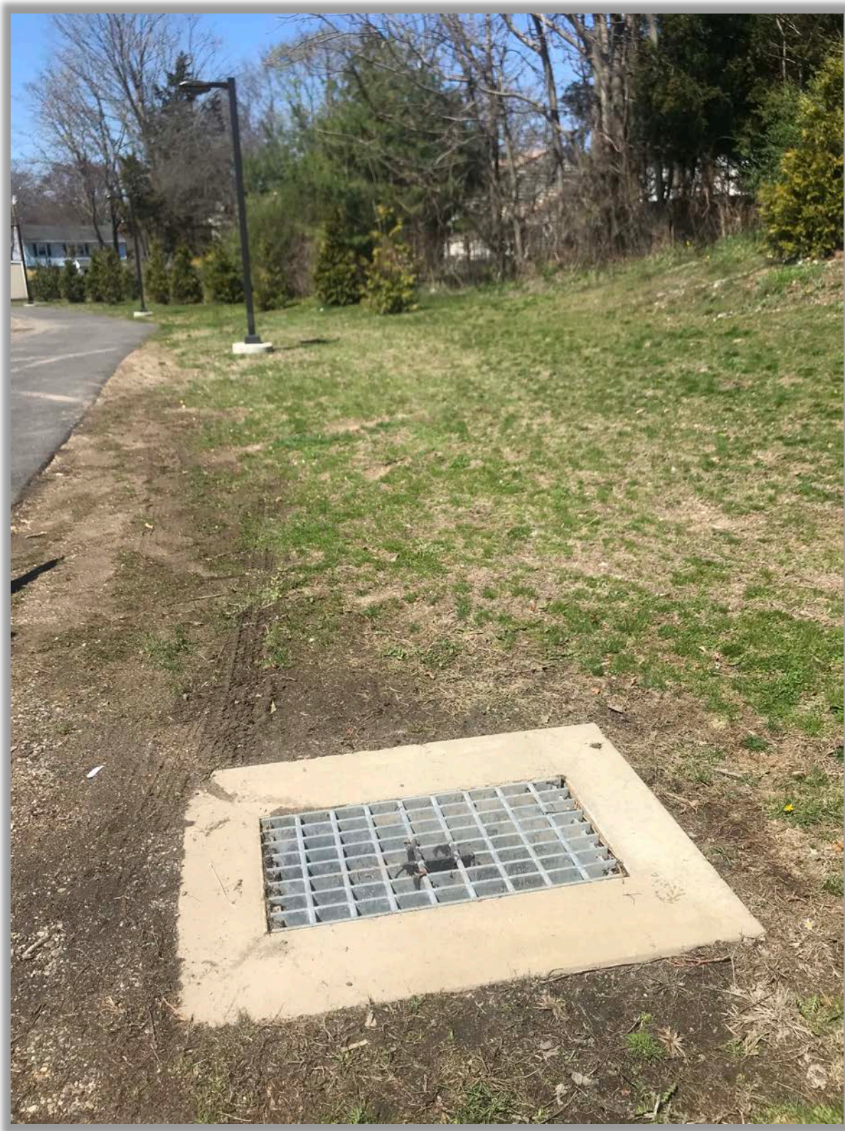
Figure 5.45: Catch basin adjacent to roadway
