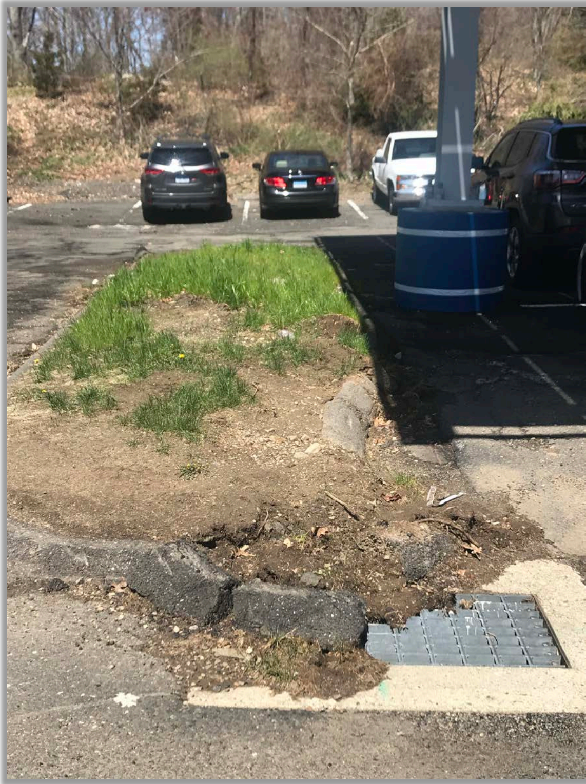
Figure 5.42: Parking lot catch basin inundated with eroding soils
