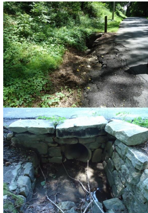
Figure 7-3. Area of Erosion and Catch Basin along Bull's Bridge Road
