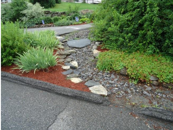
Photo 119: Rock-lined infiltration swale located off the main parking lot near the Old Building
