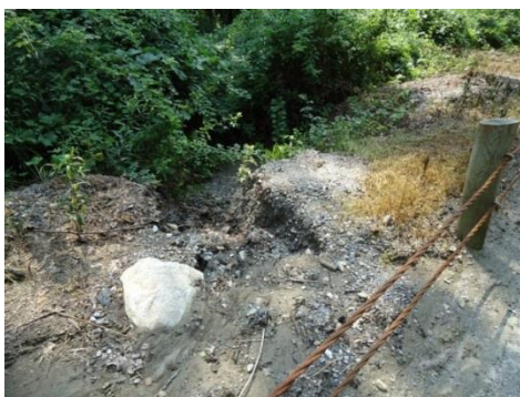
Figure 7-4. Area of Erosion along Segar Mountain Road
