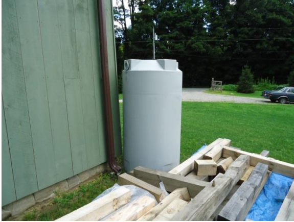
Photo 226: 250-gallon rain barrel at the Center for Innovation
