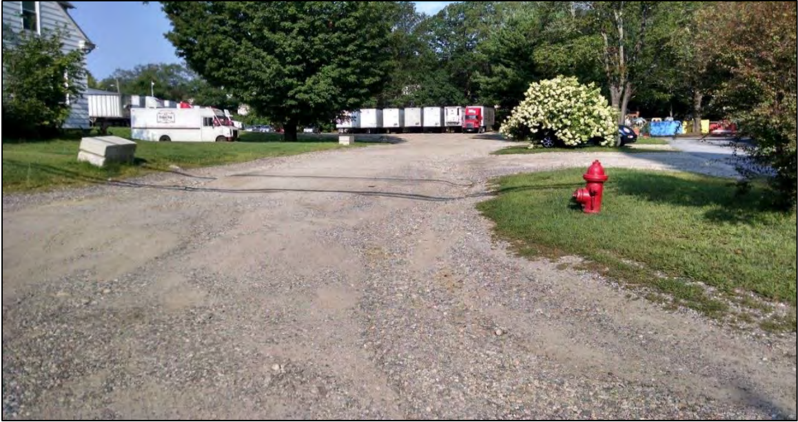
Figure 8-13. Erosion gullies formed by stormwater runoff in the Superior Bakery driveway.
