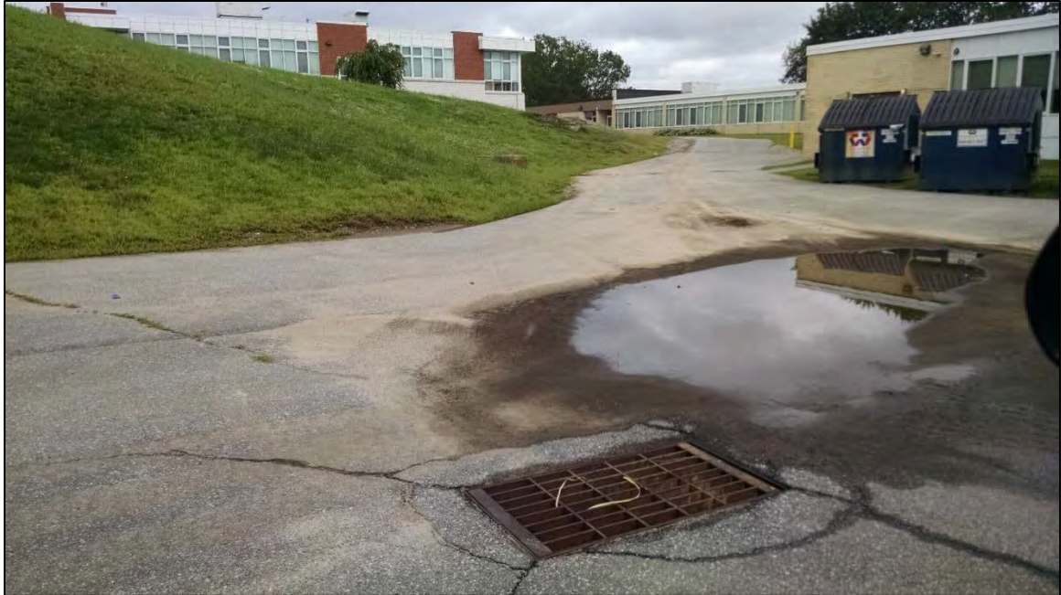
Figure 8-41. Deposition of eroded sediment near a catch basin at the school delivery area.
