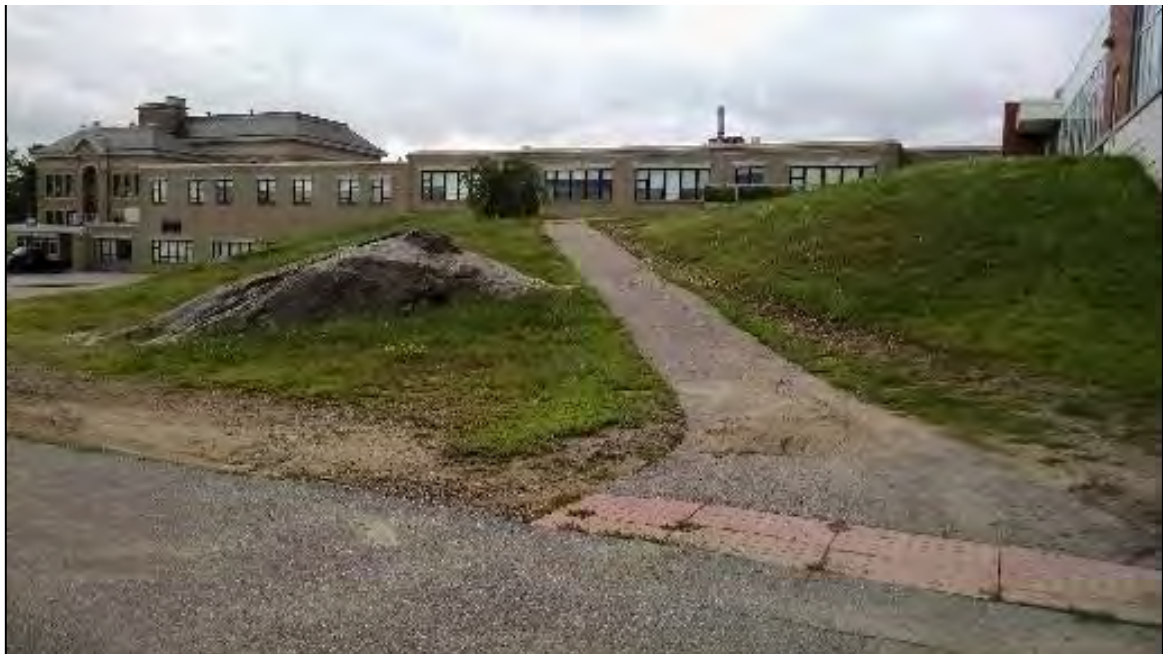
Figure 8-39. Erosion along a walkway and sediment deposition near the school delivery area.
