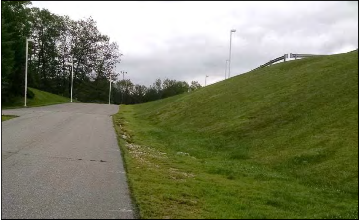
Figure 8-32. Erosion at the toe of the slope along the driveway to the high school.
