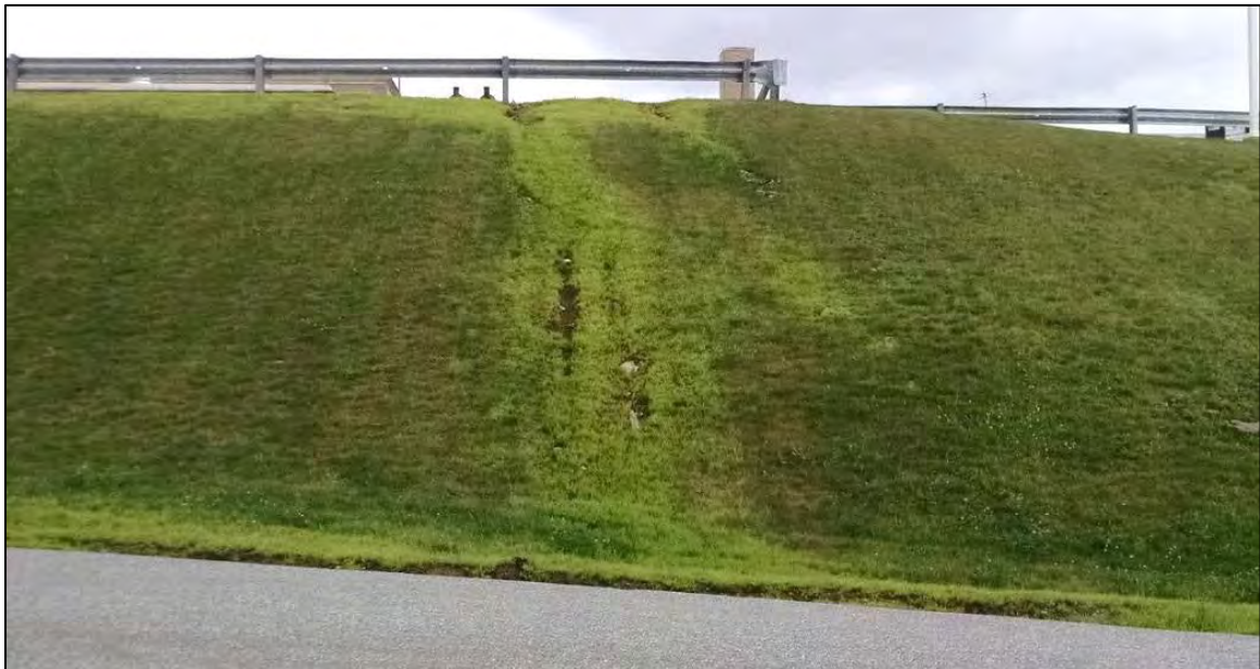
Figure 8-33. Erosion on the hillside along the driveway to the high school caused by stormwater runoff from the parking lot at the top of the slope.
