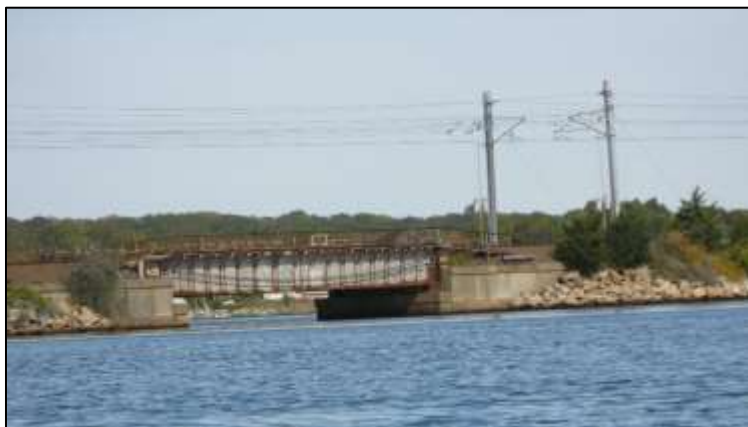
The culvert under the Amtrak rail line at the entrance to inner Wequetequock Cove.
