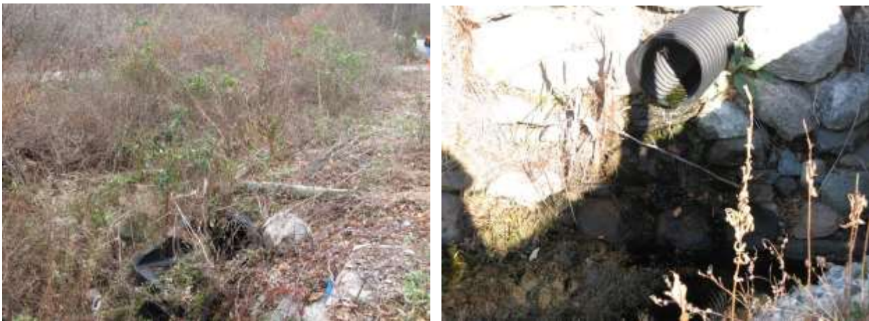
Figure 14. Stormwater outfalls from the municipal storm drain system discharged to Wheeler Brook from both the upstream and downstream sides of Taugwonk Road.
