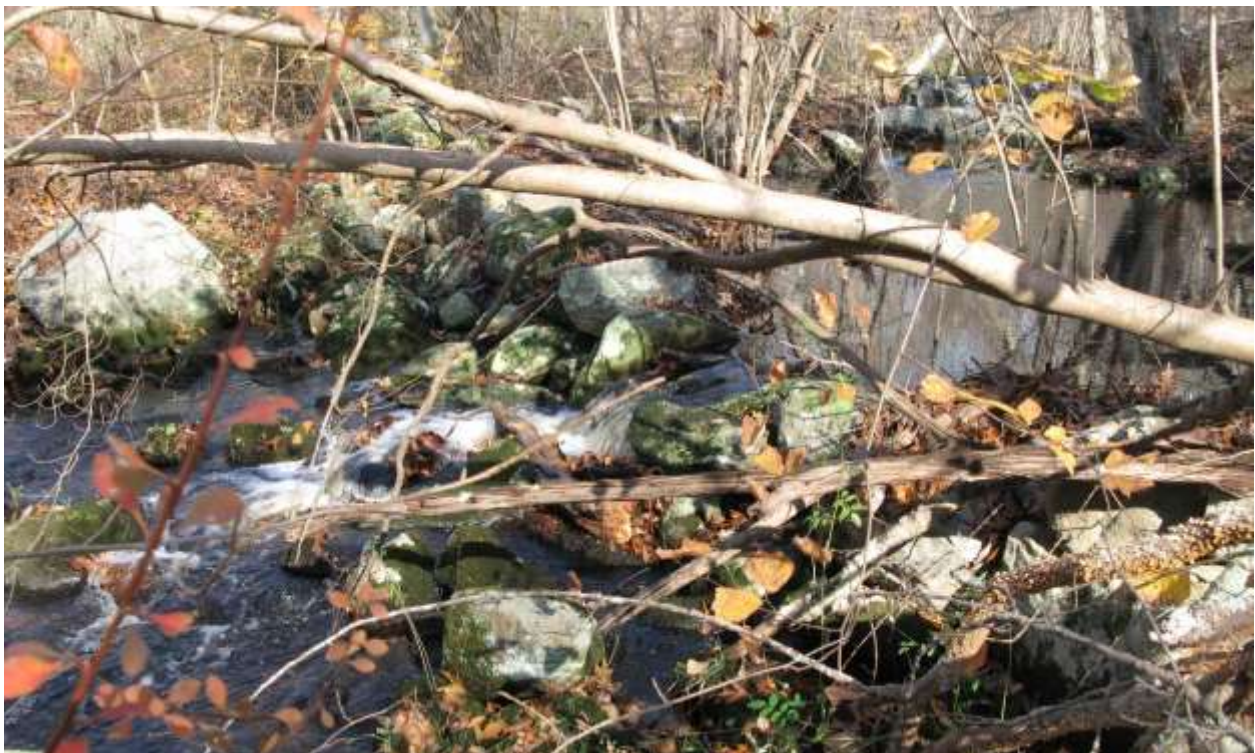
Figure 13. This stonewall built across Donahue Brook may impair fish passage particularly during periods of low flow.
