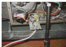
Photo 3. A gas furnace supplied by a branch circuit that has a metal gas piping system supplying it.
