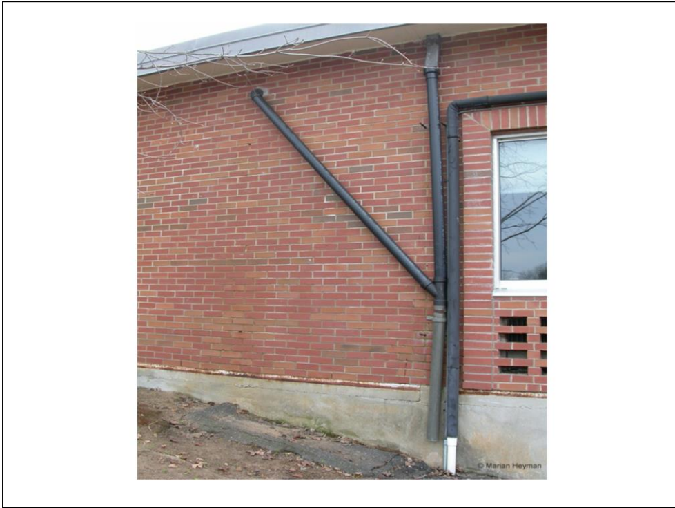
Drainage pipe (left) allowing water to drain into building.
