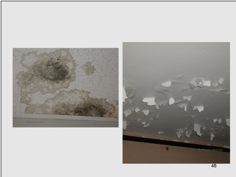
Example of chronic water problems – moldy ceiling tile, flaking paint
