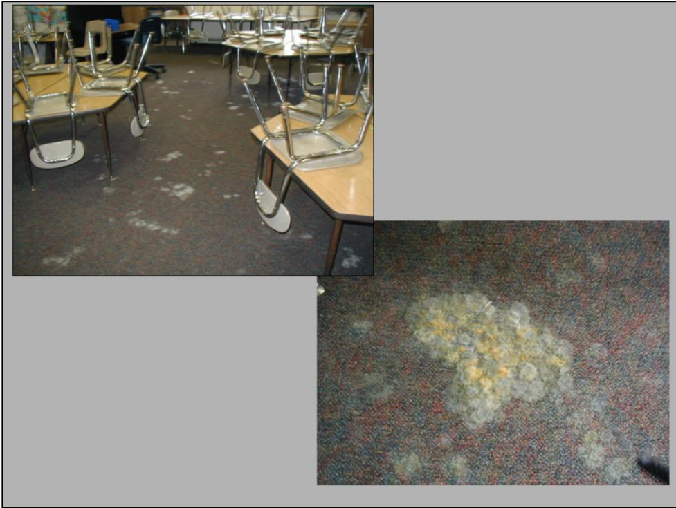
Mold growth after room shut up all summer.
