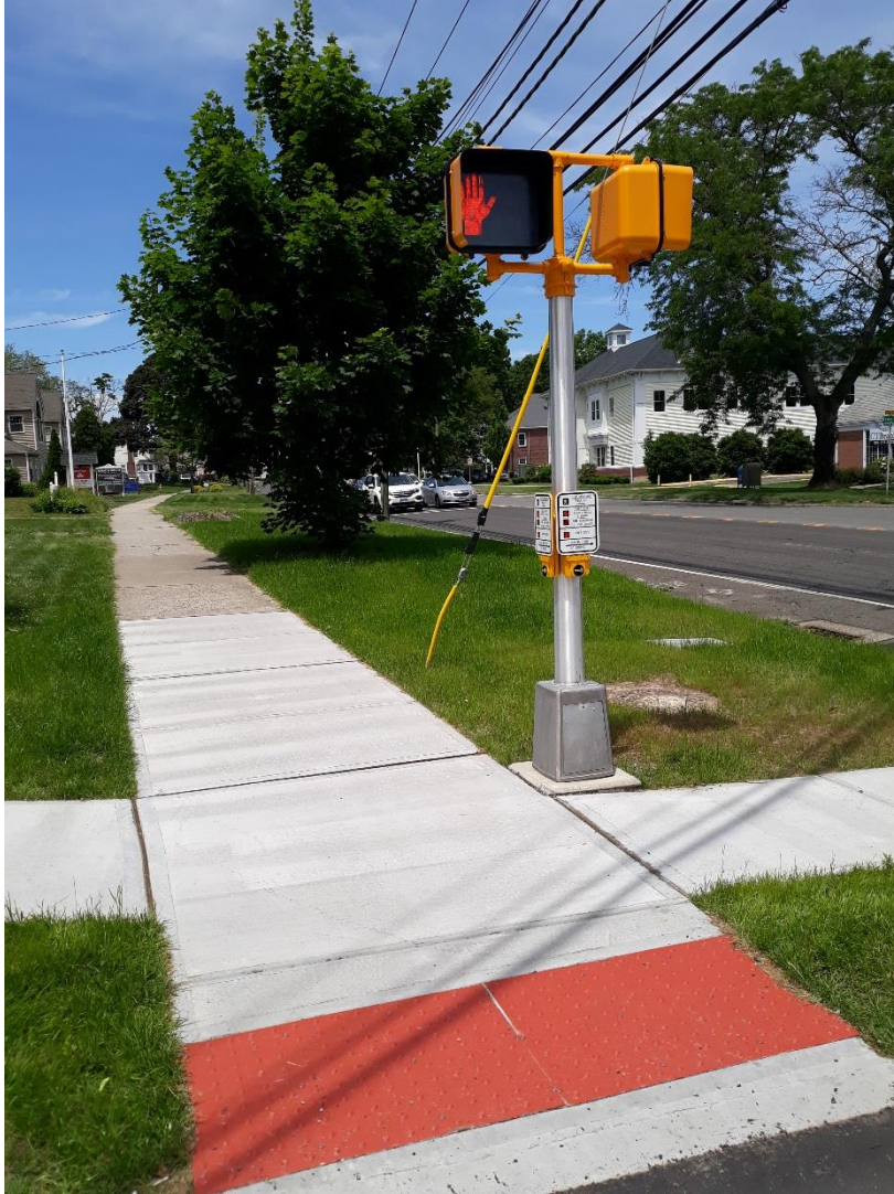
Figure 11: APS equipment at sidewalk ramp landing area
