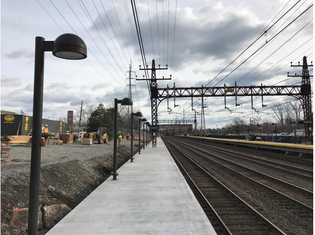
Figure 5: Noroton Heights Platform Repair (2017)
